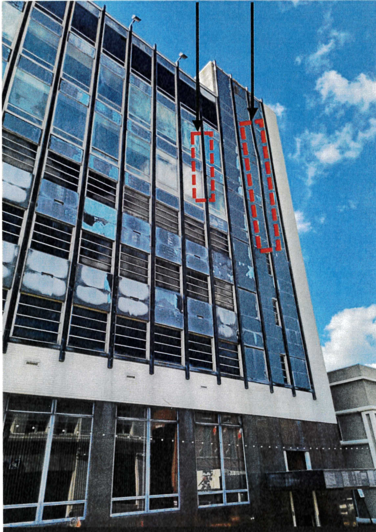
Photo 1: East Wall Elevation Showing Deflecting Wall
