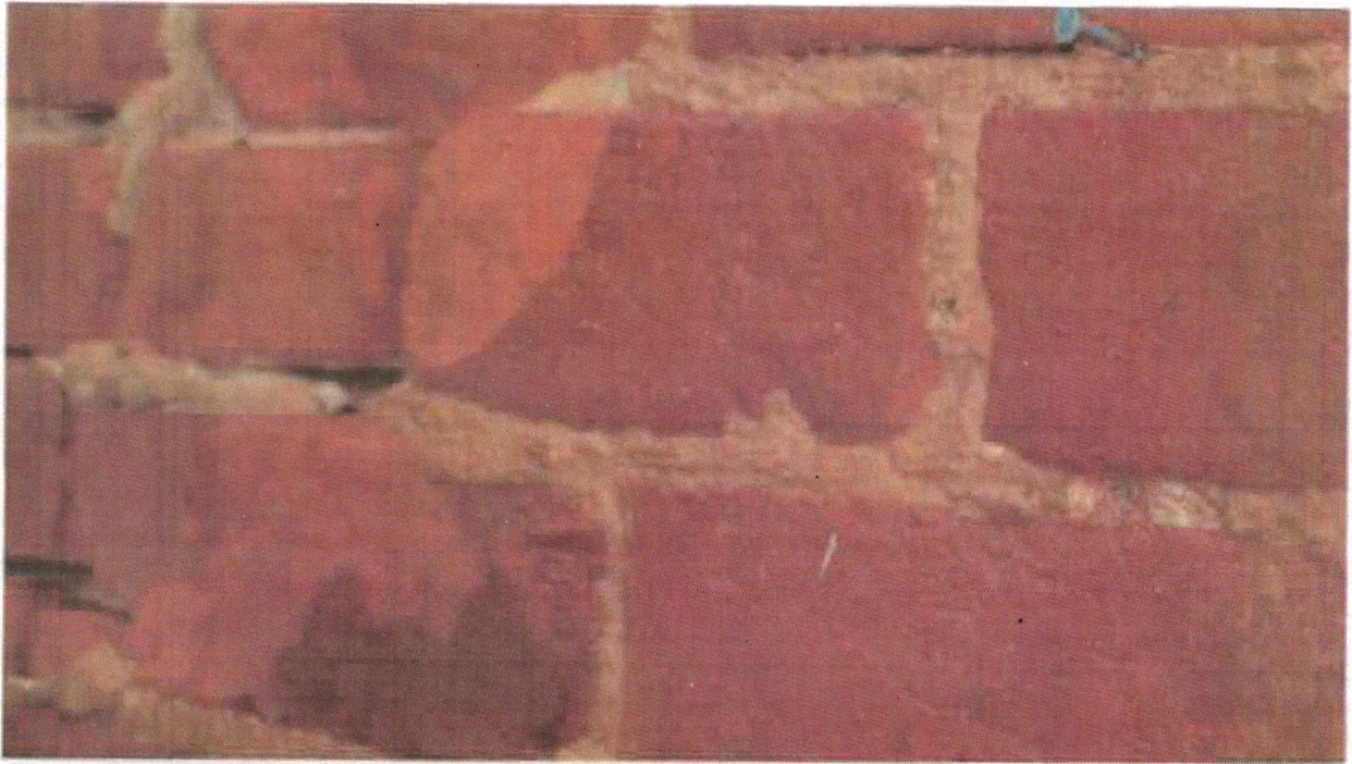
Photo 37 - Loft northeast unit looking east. Example of brick construction - sealant is evident in the darker colored brick. Where sealed the mortar is hard on the exterior of the brick, but soft 1/2" or so within the brick wall.
