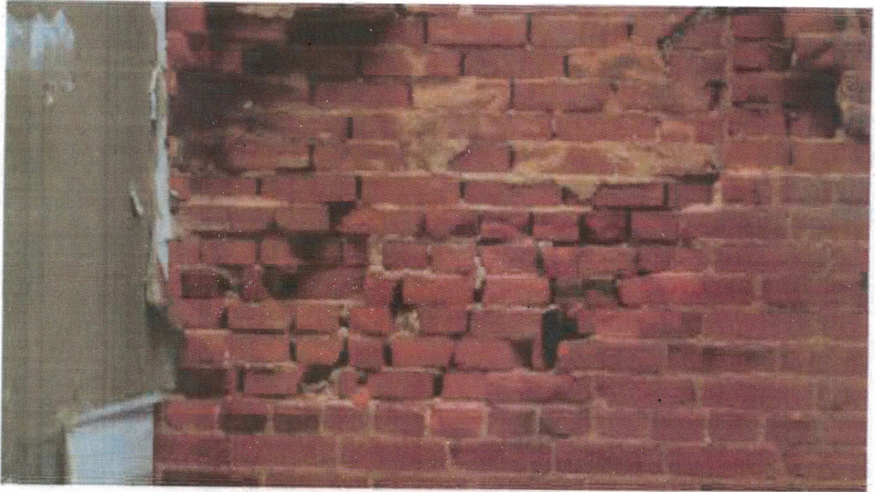
Photo 36 - Loft northeast unit looking east. Example of brick construction - missing bricks are piled on the floor not just below the bottom of this picture.
