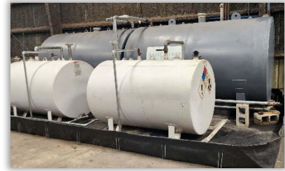
Mix Tanks and Heavy-Duty A-Frame for Filling and Servicing Machines
