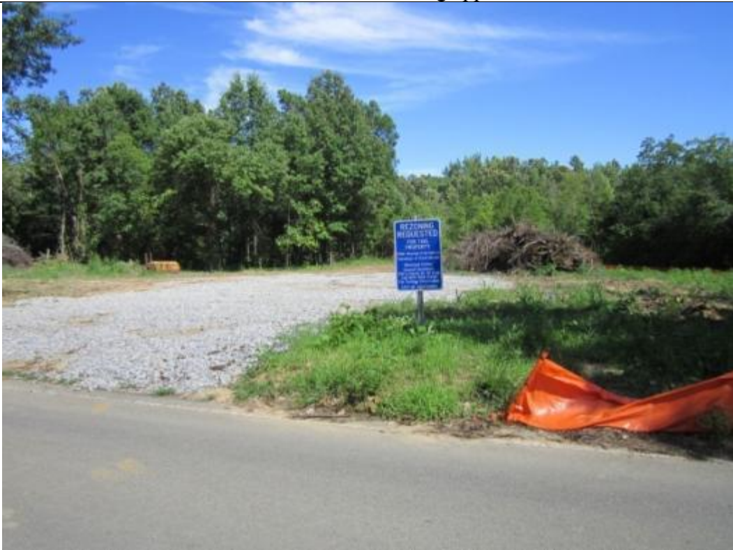
View looking south toward a construction entrance located on Greensboro Rd. that provides access to subject property.
