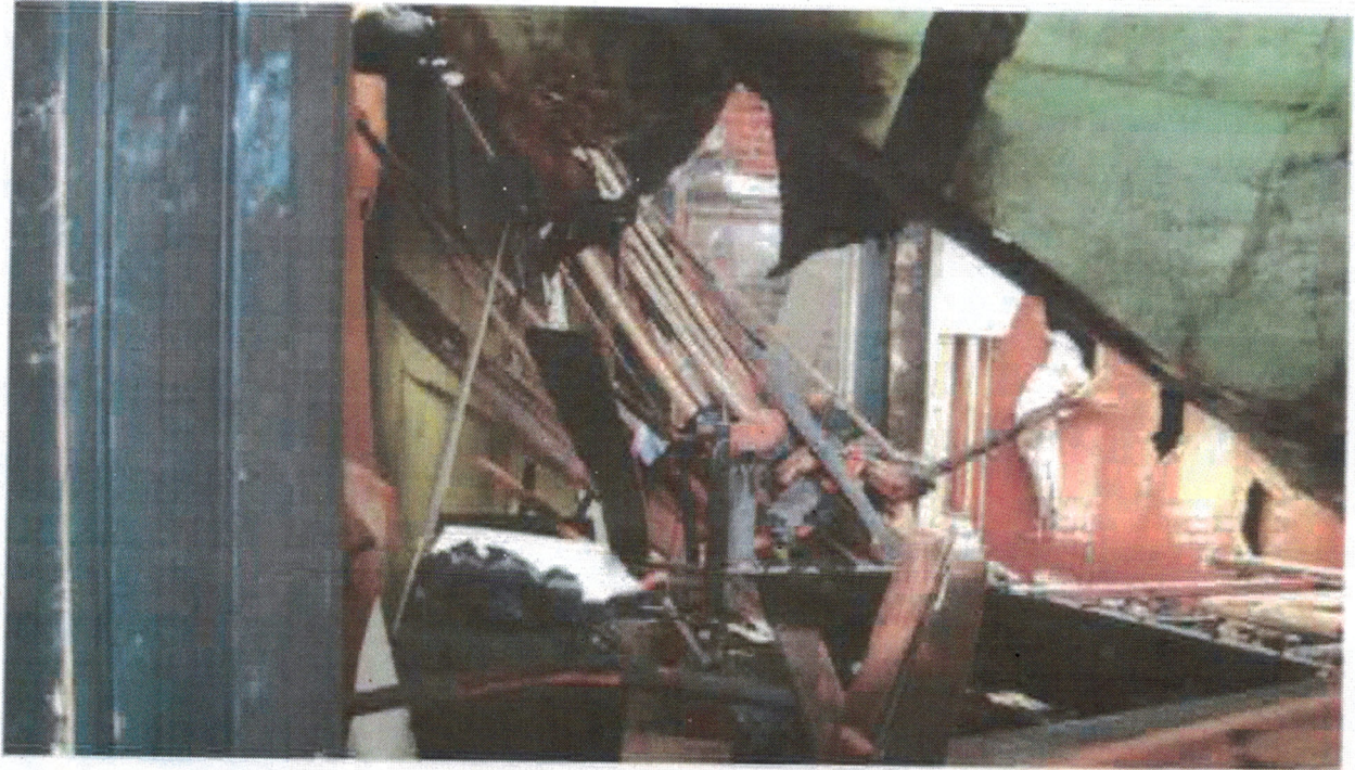
Photo 28 - Loft southwest unit. Collapsed ceiling and walls.
