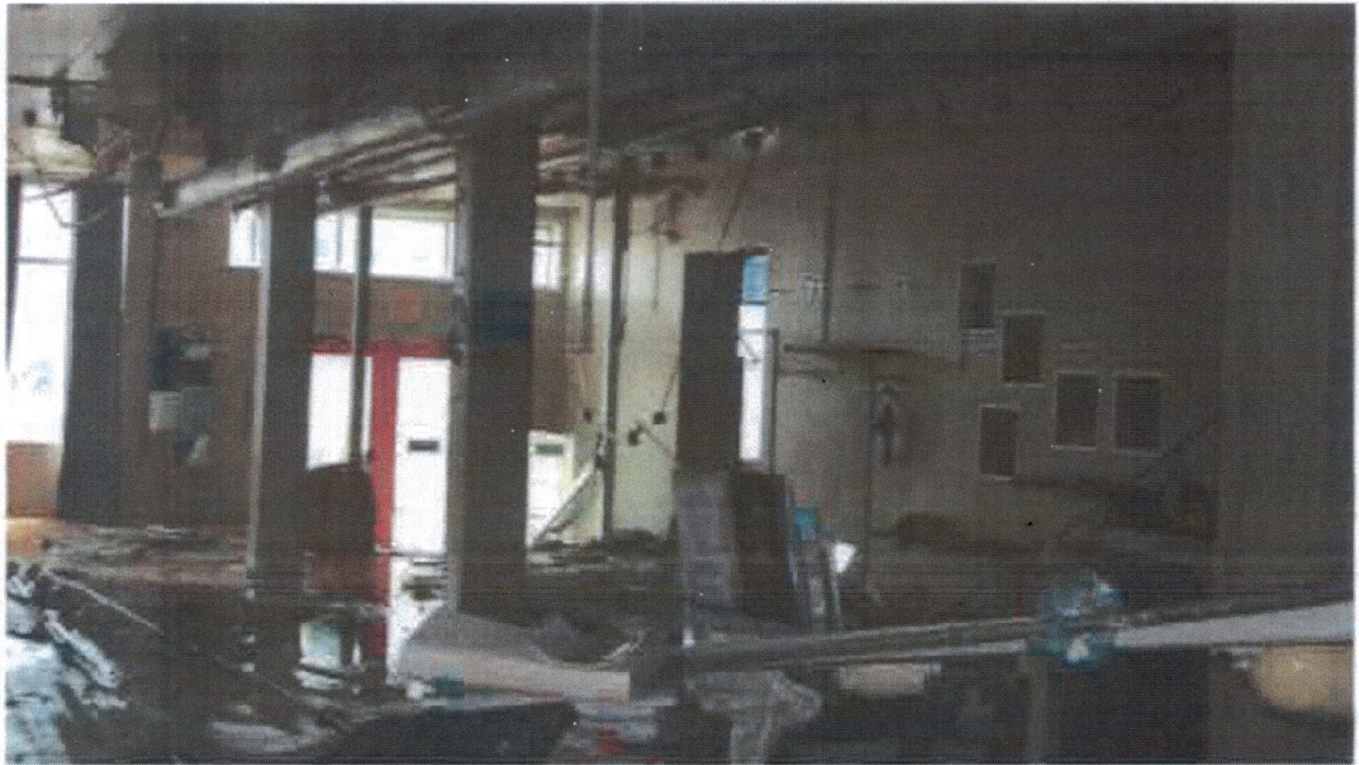
Photo 1 - Ground floor water damage to floors walls and ceiling.
