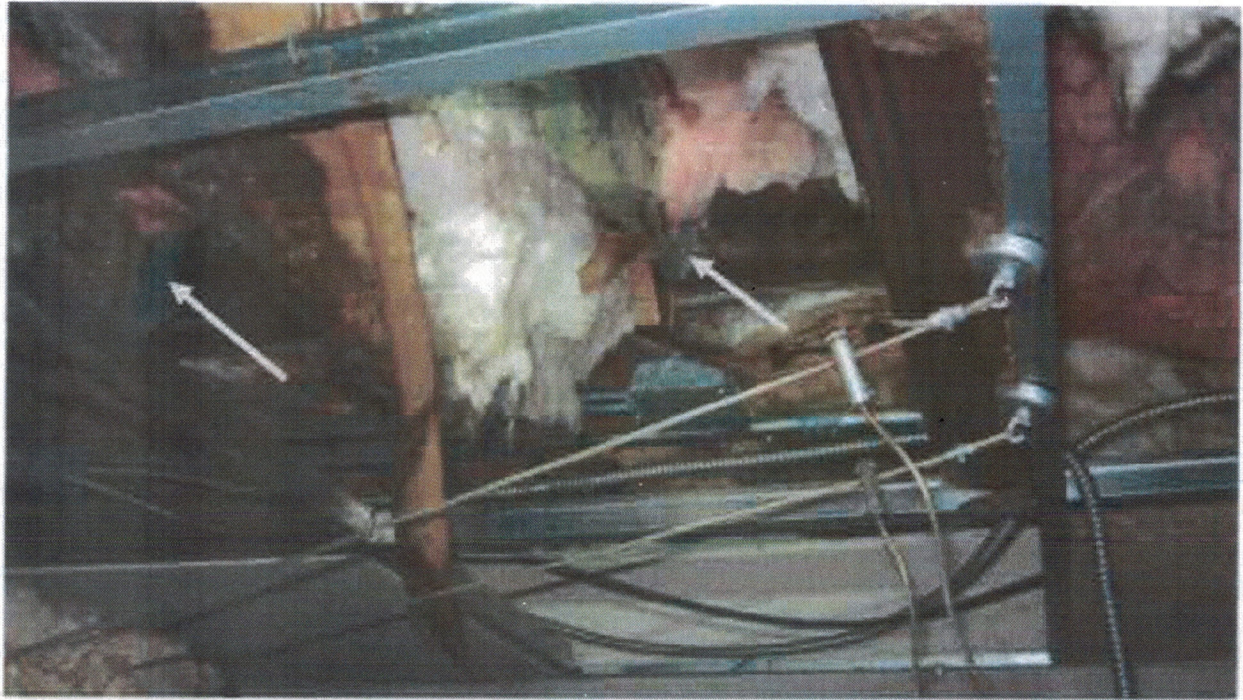
Photo 9 - Basement ceiling framing visible, see joist clips indicating a structural retrofit in the past 20-years or so.
