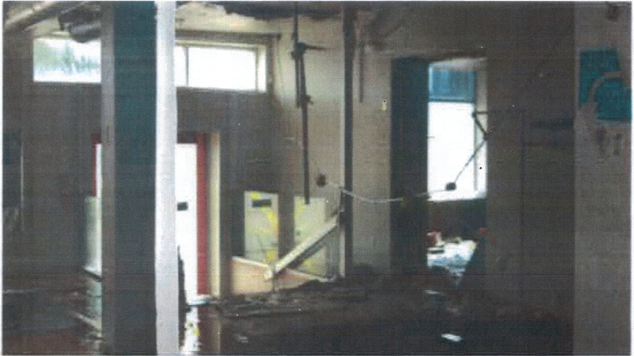
Photo 3 - Ground floor water damage to floors walls and ceiling. Conduit lost support from wetted ceiling board
