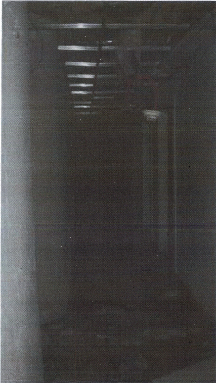
Photo 6 - Ground floor water damage to floors walls and ceiling. Mildew and mold growing on the walls.
