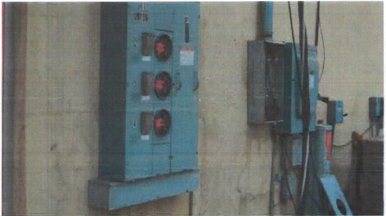
Photo 11 - West exterior wall, cracks are superficial. Electrical meter box and control boxes are undamaged.
