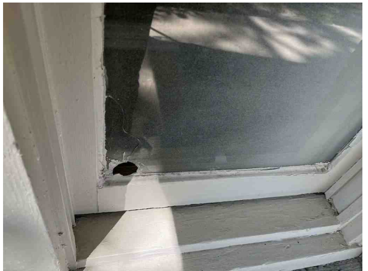
Damage to Window
