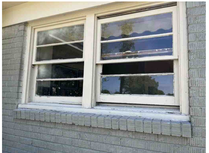
Peeling Paint around Windows
