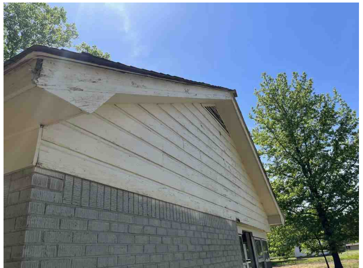
Peeling Paint along Fascia Boards
