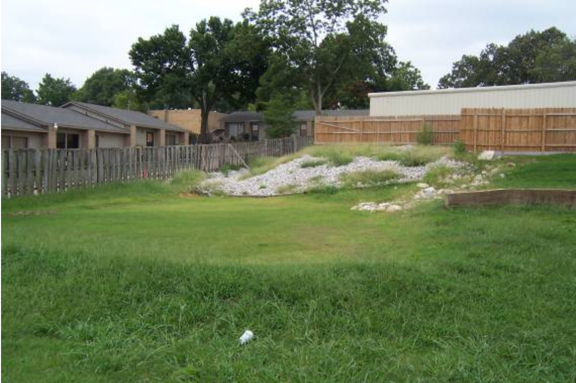
Rear of property/detention
