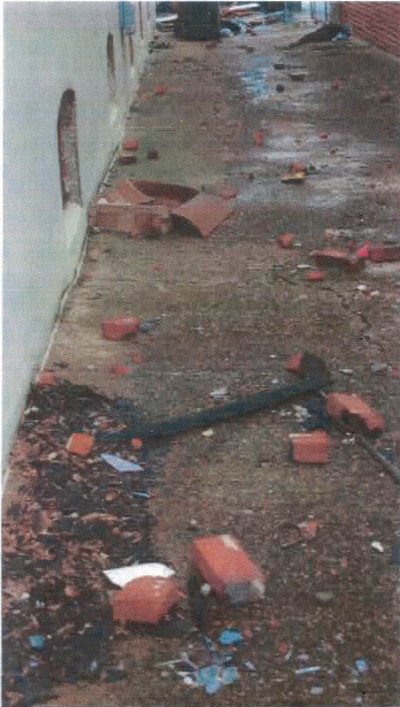
Photo 16 - North exterior wall. Fallen bricks from parapet.
