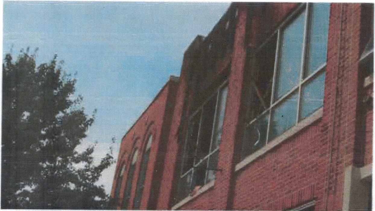
Photo 18- East exterior wall. Brick not original, or has been pointed with cement mortar. Fire blackening on parapet.
