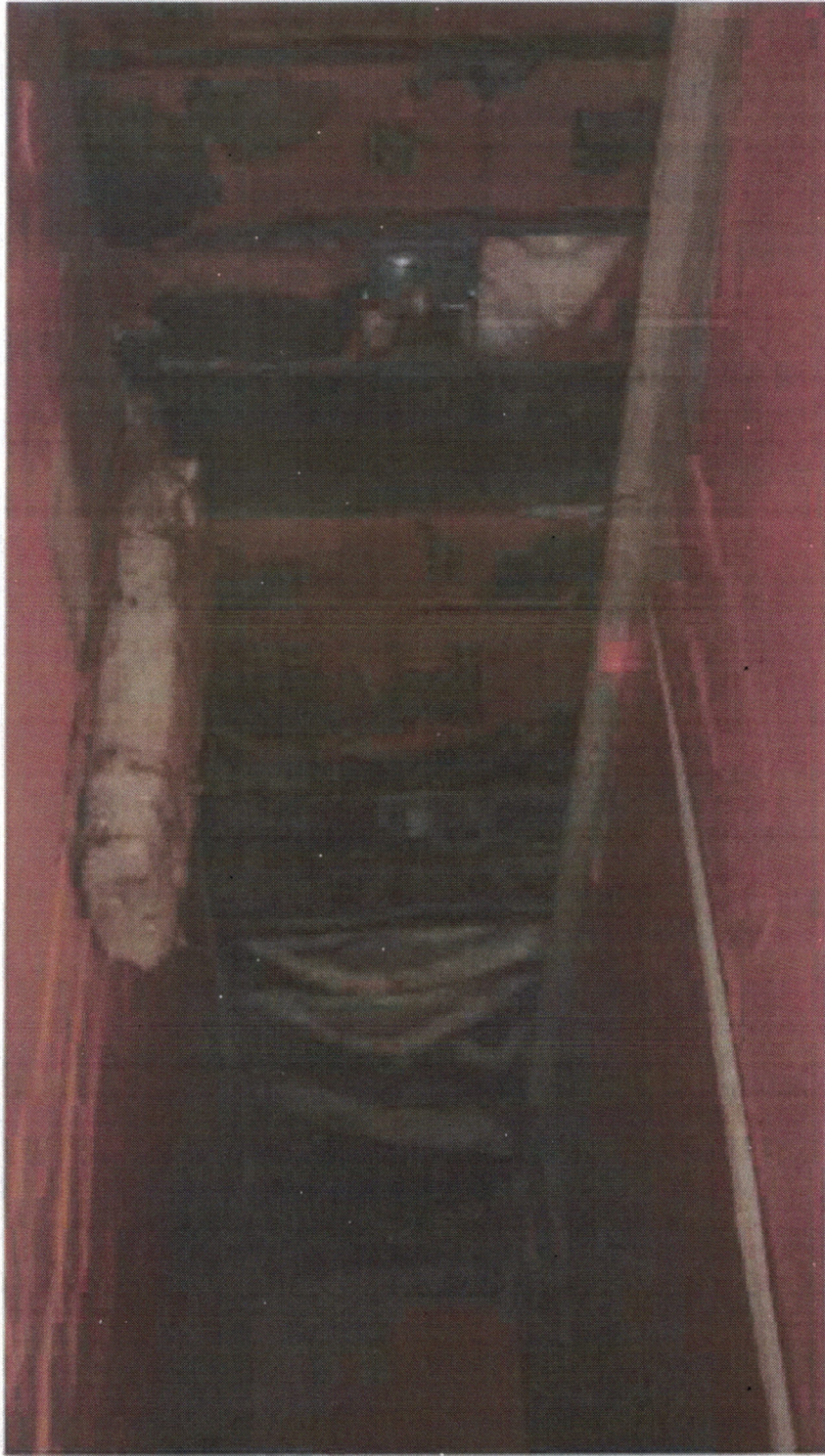
Photo 22 - stair well to 'Loft'. Water soaked gypsum board.
