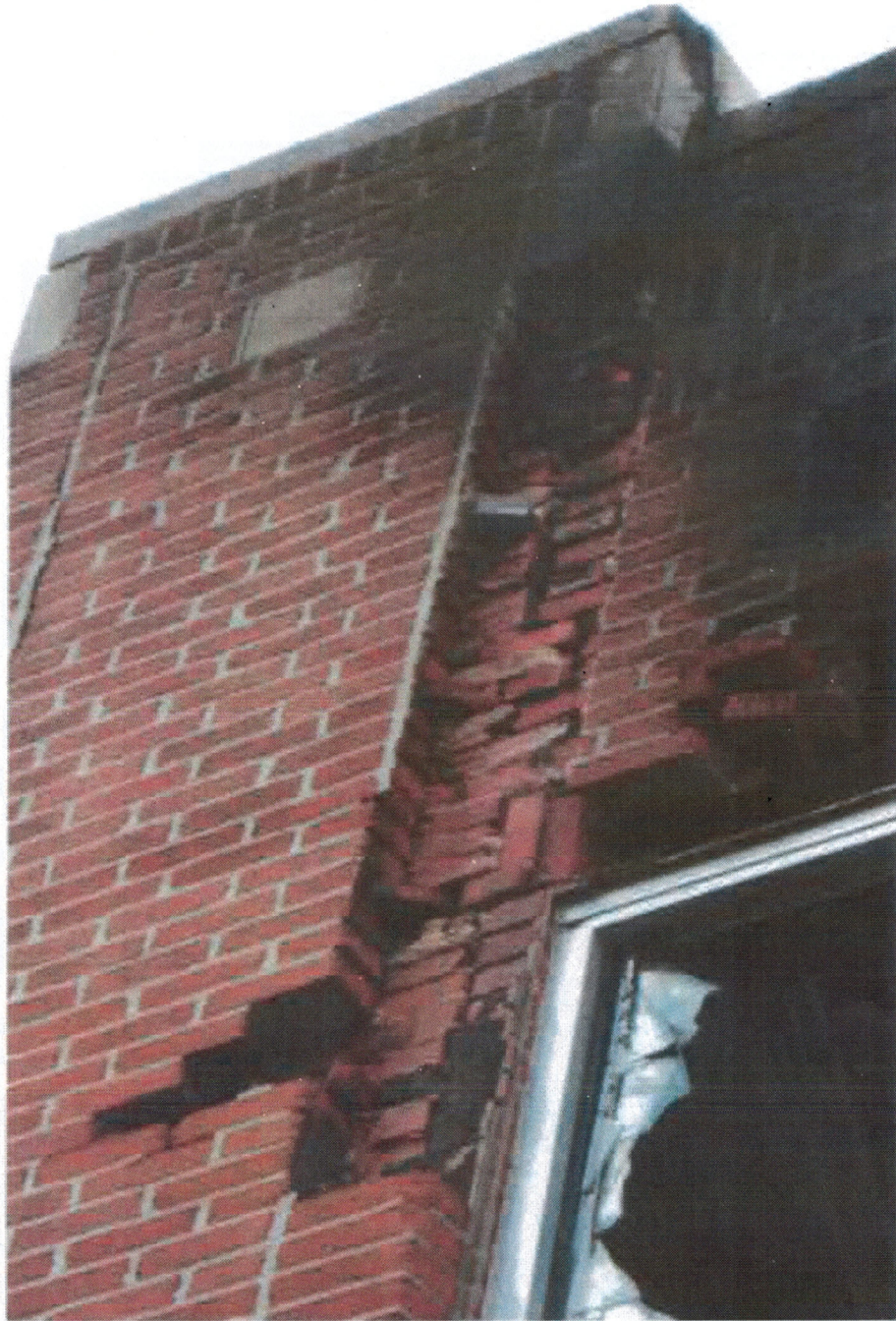
Photo 21 - East exterior wall. Brick not original, or has been pointed with cement mortar. Brick is stacked and not properly bonded with mortared or not tied with soldier course.
