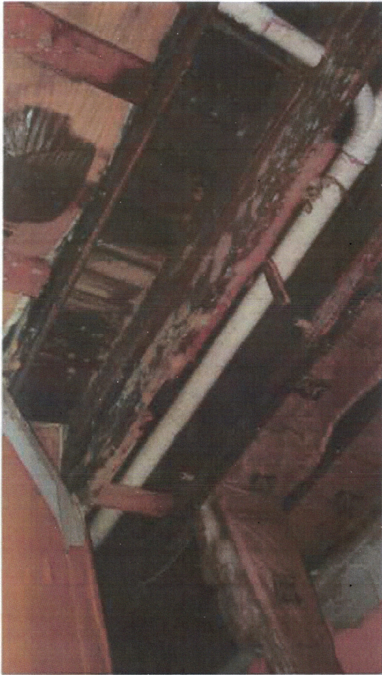
Photo 23 - Ceiling in stairwell. Gypsum board and insulation water soaked
