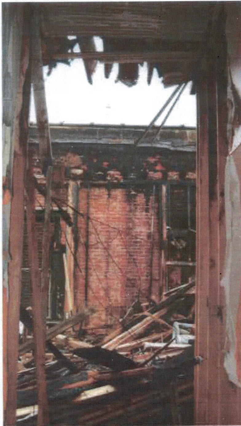
Photo 26 - Loft looking south. Ceiling consumed by fire and collapsed onto floor. Windows look into light well formed by adjoining building.
