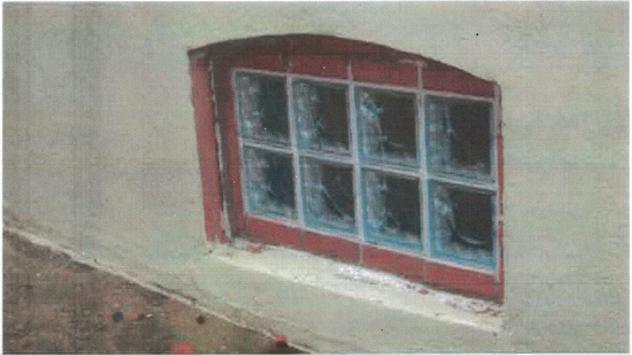
Photo 15 - North exterior wall. Broken glass block.
