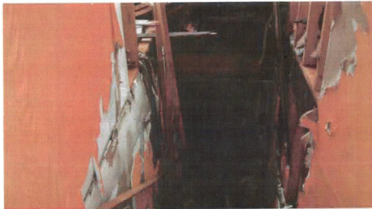
Photo 25 - Ceiling in stairwell. Gypsum board and insulation water soaked
